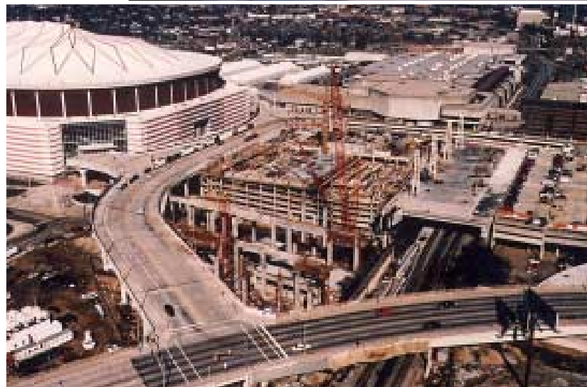
The Georgia International Plaza for the 1996 Olympics in Atlanta was constructed above a multi-level deck in a heavily congested area.
